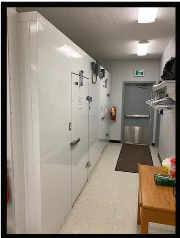
Walk-in Fridge & Freezer & South Door
